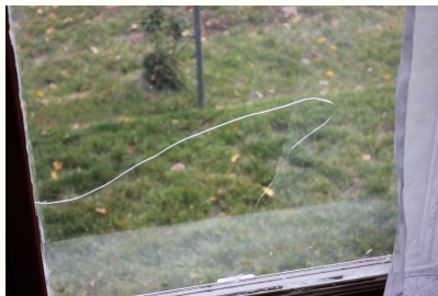
One of two broken window panes observed.
