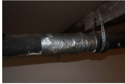
This pipe appears to have an improper repair to it, and is not properly supported.
