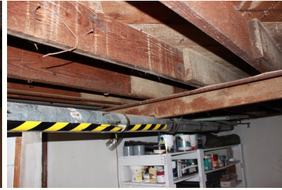
These sections of the drain waste pipe appear to have been improperly repaired with sheet metal duct pipes and sealant.
