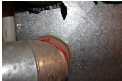
The red tape in this picture is not of the type typically used to seal duct joints.
