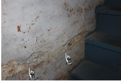
Vertical crack in foundation most likely caused by water penetration and negative grade to the outside wall. The sidewalk in this area has been replaced recently and the grade issue has been corrected.
