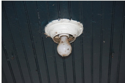
This light is located on the front porch and should have a proper weather protective globe cover installed on it.
