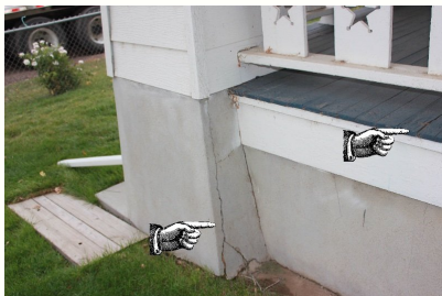
Cracking in front porch column. Wood deterioration on front porch decking.
