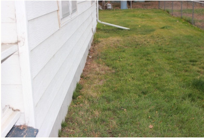
This is the west side of the home. The grade slopes towards the foundation and there is a small trough area next to the foundation that can pool water.
