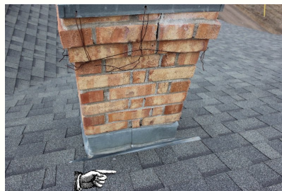
This side of the chimney should have cricket flashing installed to divert the water around the structure.
