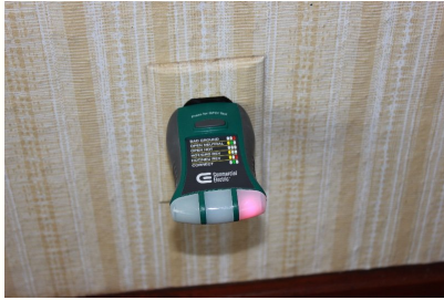
One of several outlets that has a bad ground.
