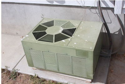
Existing central air unit.
