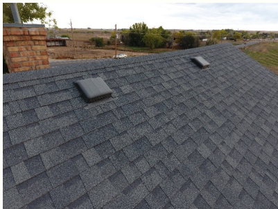
roof shingles and vents on the south back side of the home.
