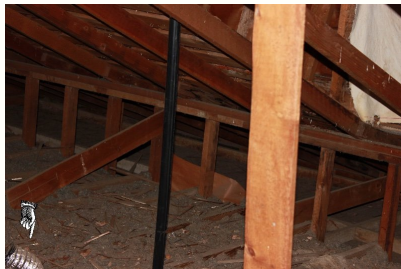
Improper termination of bathroom vent in attic.
