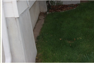
Negative grade at front porch supporting wall.
