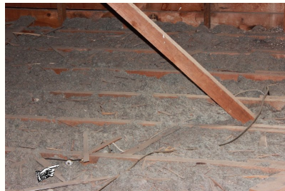
More knob and tube wiring improperly installed in the attic.
