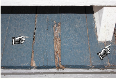
Wood deterioration on front porch decking.
