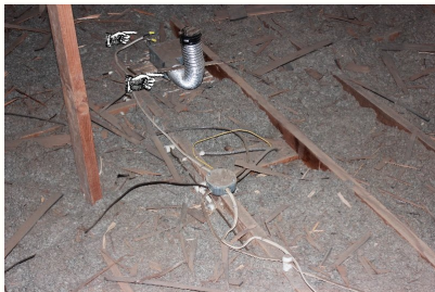
Improper termination of bathroom fan, wiring splice is not properly contained in an approved covered box.
