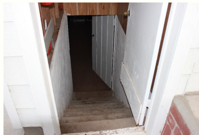
Basement access door from the backyard improperly opens over the stairs. This is a safety hazard and the door needs to be reversed to swing outwards. The door is not designed for exterior use and thus is deteriorating and should be replaced at the same time.
