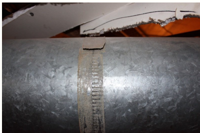
Another joint that needs repaired with new tape.
