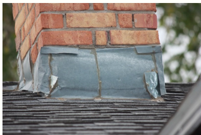
Improperly installed flashing at base of chimney on roof.
