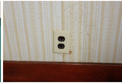
One of several outlets that is not properly grounded.
