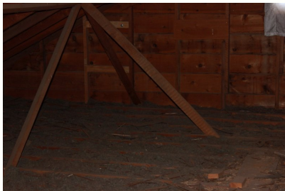
These roof supports should be checked and verified by a structural engineer as properly installed.
