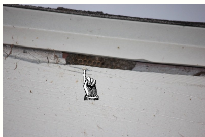
Evidence of wasp infestation in the eave rake on the north east front of the home.
