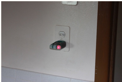
Electrical outlet showing a bad ground on outlet tester, also needs to be upgraded to GFCI outlet.
