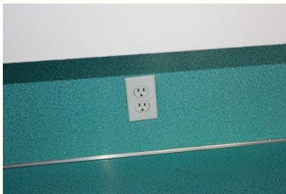
Non GFCI outlet in the kitchen.
