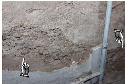
Continuation of the crack.
