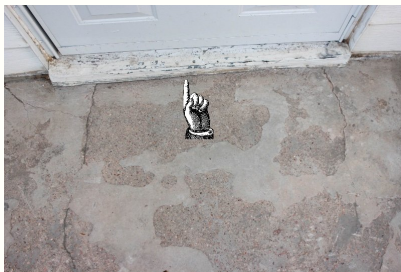
Wood deterioration on back door leading to the main floor.
