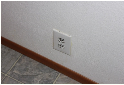
Electrical Outlet in master bathroom needs removed or upgraded to GFCI receptacle.
