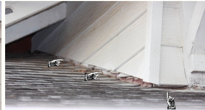
This area appears to be not properly flashed. the siding is installed correctly, and there may be over a brick. Even if the brick is considered water tight, because of the nature of the different material intersecting, flashing should be installed. A licensed contractor should be contacted for further evaluation and pricing.
