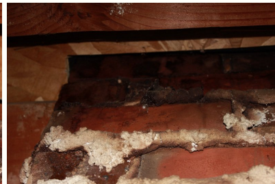
Brick chimney stack in attic showing improper repair to deteriorating mortar joints.
