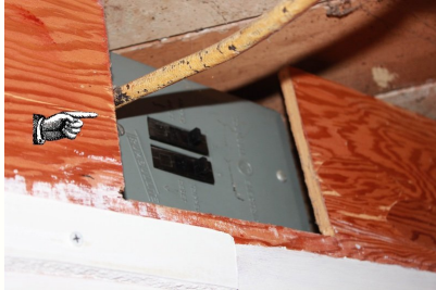
This sub-panel located in the basement rafters is not in a proper location.
