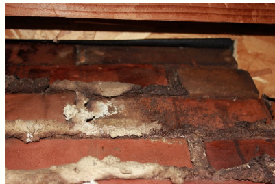
mortar joints on chimney stack in the attic showing deterioration. efflorescence is also present indicating past water damage.
