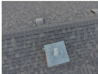
roof shingles from drone picture, viewing above chimney and peak of roof.
