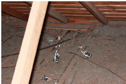
Antiquated knob and tube wiring improperly installed. This is a serious concern and should be examined and upgraded by a licensed electrician as soon as possible.
