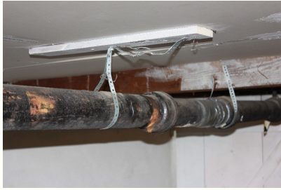
Improperly supported cast iron drain pipes.
