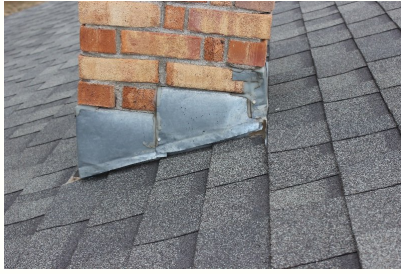
Improperly installed step flashing.
