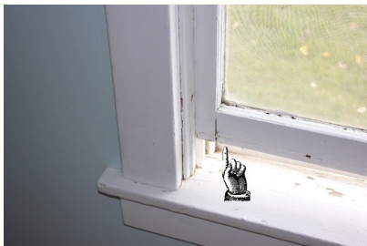
Wood deterioration can be observed on the sash of this window.
