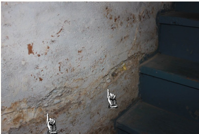
This crack in the east wall should be monitored moving forward.
