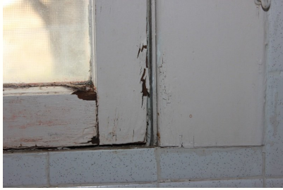
Water damage to the window sash and frame.
