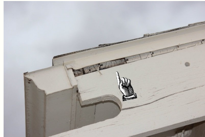
Improperly installed flashing, the flashing length is not sufficient to cover the gap, thus allowing water penetration.
