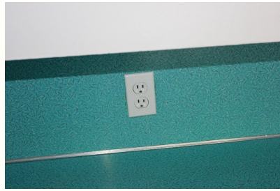
Electrical outlet in the kitchen needs upgraded to GFCI receptacle.
