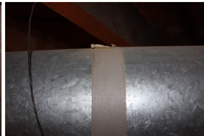
The old tape on this duct joint has deteriorated and needs removed and replaced.
