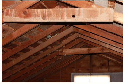
Roof frame showing OSB sheathing over former roof battens, supported by 2"x6" roof rafters. Two collar beams can also be seen adding support to the rafters.
