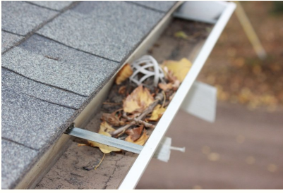
Debris and sediment build up in the gutters on the roof.
