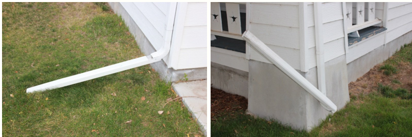
Downspout extension should be extended out further to a minimum of 6' or more from the foundation.
