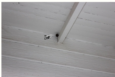
Wasp nest @ exterior wall and soffit corner.
