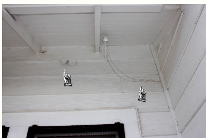
Wiring not properly installed within an approved box with cover, and abandoned wires.
