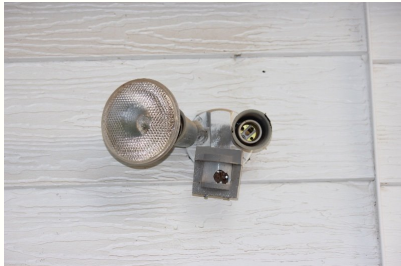
This light is missing a bulb and it appears the motion sensor may be broken. A licensed contractor should be consulted for repair or replacement.
