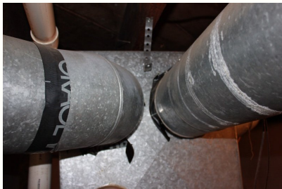
The sealant tape is begging to pull lose from the joints around the furnace and ductwork.
