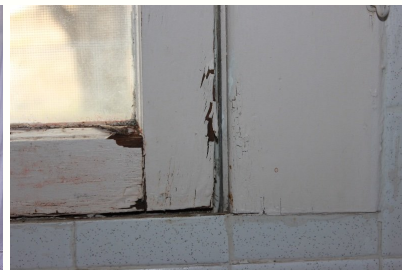
The wood on the sash of this bathroom window is rotting from excessive water penetration.
