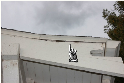
Flashing should properly extend over this gap and sufficiently onto the 2"x8" outer roof rafter below it.
