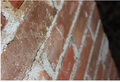
Chimney stack with deteriorating and improperly repaired mortar joints.
