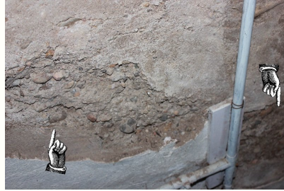
Vertical crack continues into the main room of the basement.
