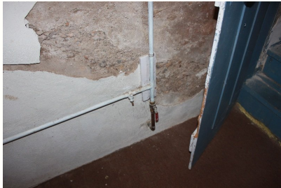
Water entrance and interior supply shut off in the basement on the east.
