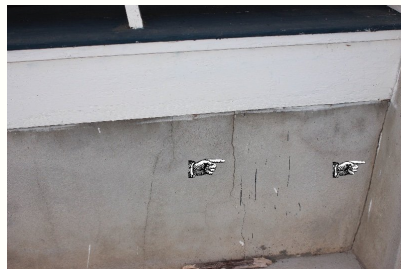
Cracks in front supporting wall, and separation crack in column.
