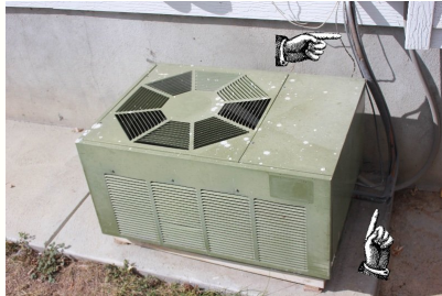
The supply and return lines need new insulation wrap.
