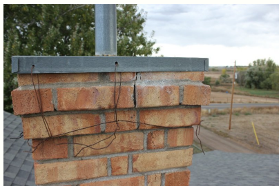
Rain cap improperly secured to chimney. Mortar failure and cracking in the brick joints.
