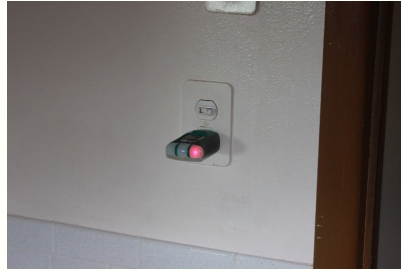
Electrical outlet in the hallway bathroom, bad ground and no GFCI.
