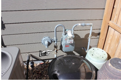
Gas meter, the finger points to the main shut off for the house.
