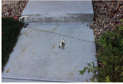
The sidewalk to the front door has a settling crack and efflorescence stains that may indicate drainage problems..
