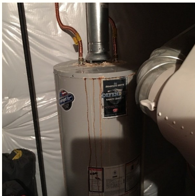
Hot water tank showing signs of past leak and rust.. Heavy mineral buildup / efflorescence can be observed on the top and in the pan below.
