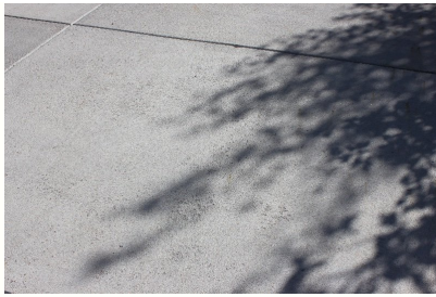
The spalling seen here will continue to worsen with the freeze thaw cycle of the local climate.
