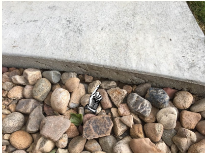
The grade is eroding on this side of the sidewalk that leads to the back yard. It should be built up to prevent further erosion and problems.
