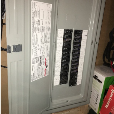
Sub panel with all circuits labeled.
