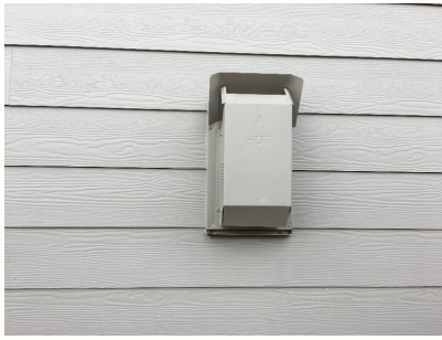
Metal flue for living room gas fireplace on the east side of the home.
