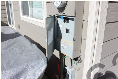
This main panel door does not properly open without removing the hot tub cover.
