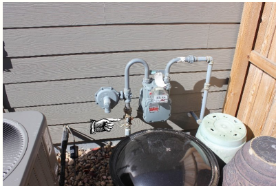
Gas meter located in the back yard on the east side. The hand in the picture is pointing at the main shut off valve for the house.
