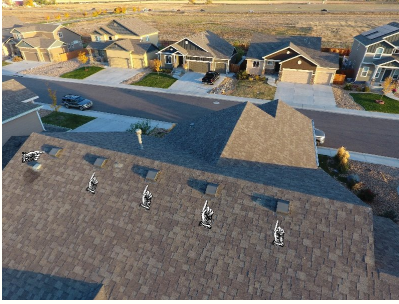
Drone picture of roof, fingers pointing at the ridge vents for the attic.
