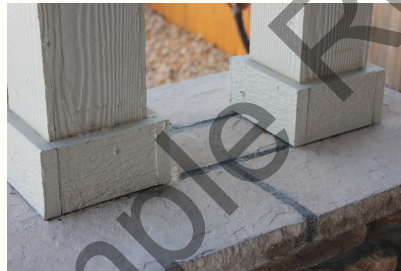
The base of these columns should be caulked to prevent water penetration.
